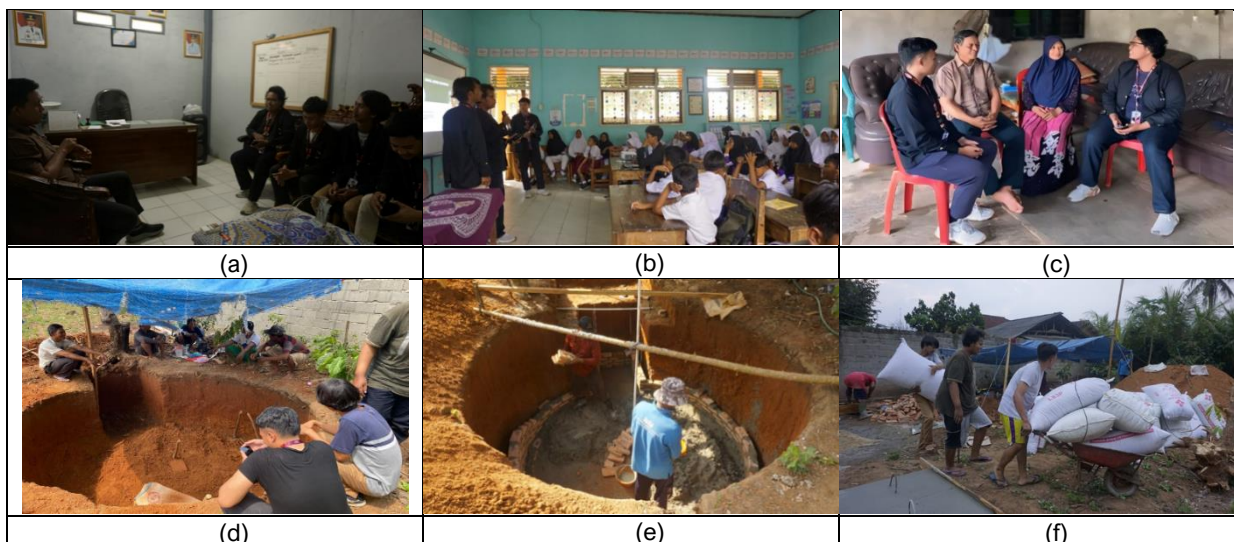
FIGURE 3. (a) Visit Stages Before Reactor Construction Project, (b) Socialization of SDN 2 Labuan Ratu Satu, (c) Socialization to Cow Shed Owners, (d) Digging a Hole for the Reactor, (e) Reactor Installation Process, (f) Community and Team Participation in Reactor Construction
