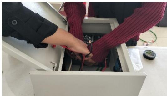
FIGURE 6. Solar panel system assembly (Source: Author's, 2024)
