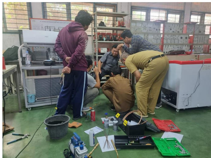
FIGURE 2. BLK Instructors in Karawang Regency are preparing for the practical session on replacing refrigerant from R410A with R290 in split AC units.
