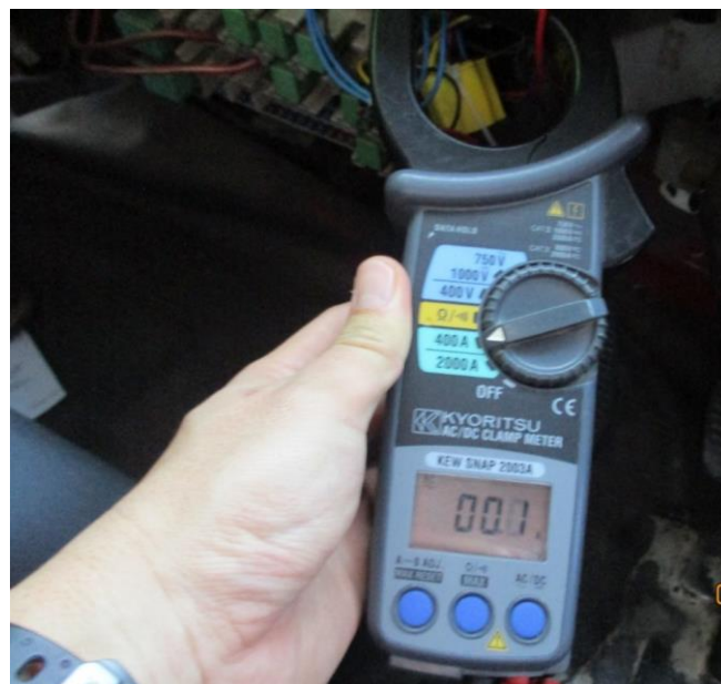
FIGURE 6. Results of leakage current testing on the ESI tool
