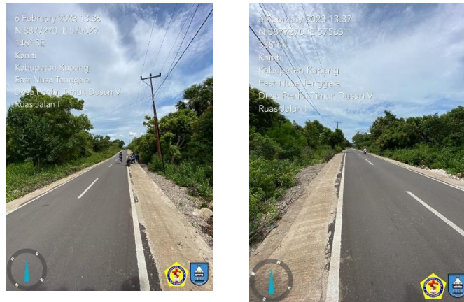
Figure 2. Roads Condition in District V of Penfui Timur Village
