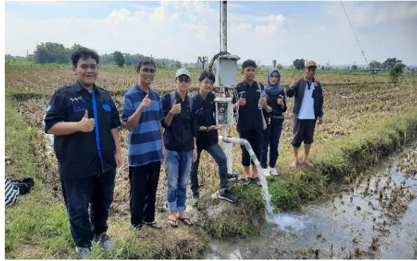
Figure 9. The installed device works properly
