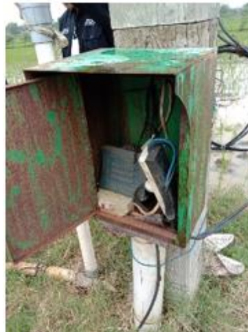
Figure 4. Poor old switching unit condition
