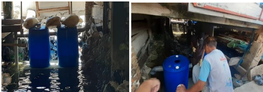
Figure 8. Installation of latrines in the columns of residents' houses which are inundated by sea water
