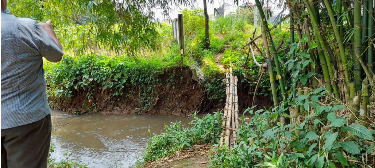
Figure 3: Survey of the location of the pedestrian bridge with a bamboo base
